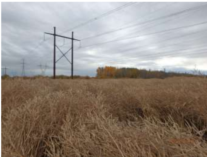
THE COMPLETED LINE
